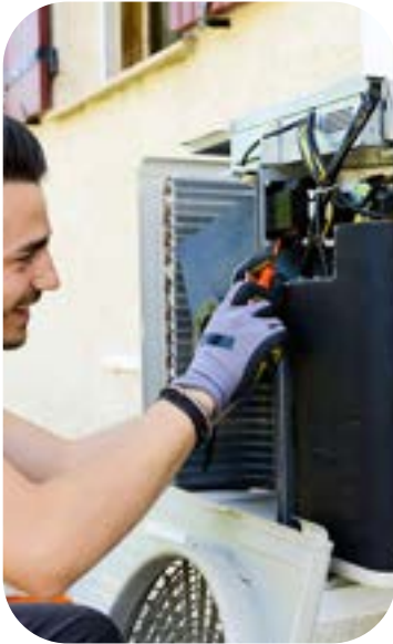
Air-conditions, ventilation & air filtration system & maintenance.
