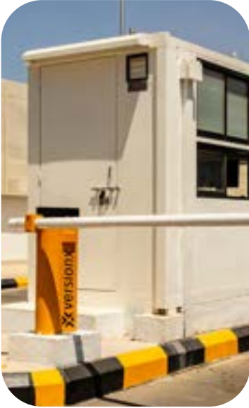
Parking Management Electronic systems installation & Maintenance
